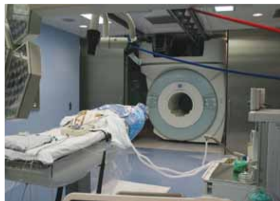
The steel doors opens and the magnet moves towards the patient on rails installed in the ceiling
